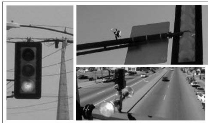
Traffic Signal Mast Detector and Indicator Light
